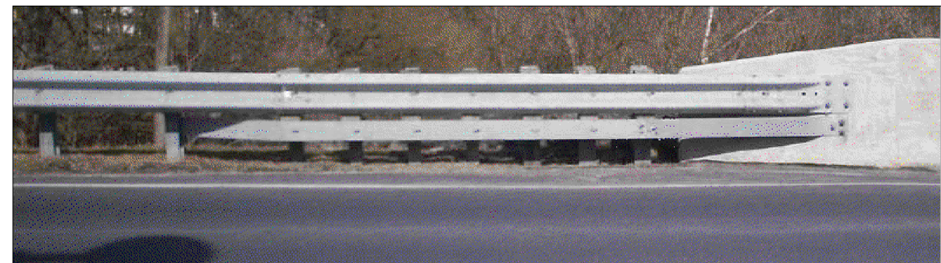
ELEVATION VIEW FOR TYPICAL CONCRETE BRIDGE BARRIER TRANSITION (WITHOUT INLET PLACEMENT) FOR DETAILS, SEE SHEET 1
