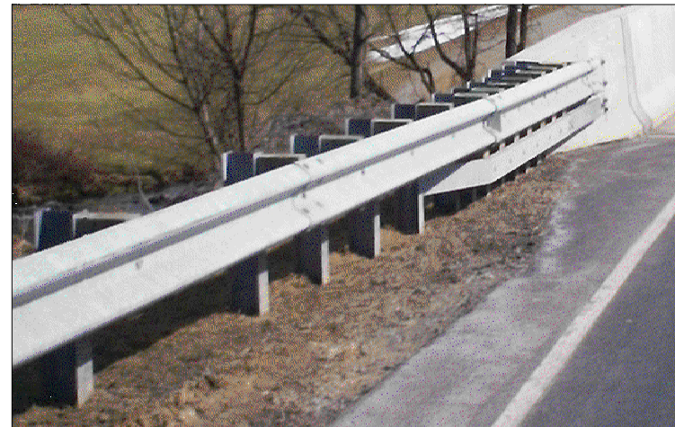
GUIDE RAIL TO TYPICAL CONCRETE BRIDGE BARRIER TRANSITION (WITHOUT INLET PLACEMENT) FOR DETAILS, SEE SHEET 1
